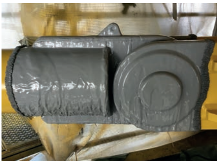
Catlink Transverter Station courtesy PeperEnergy
