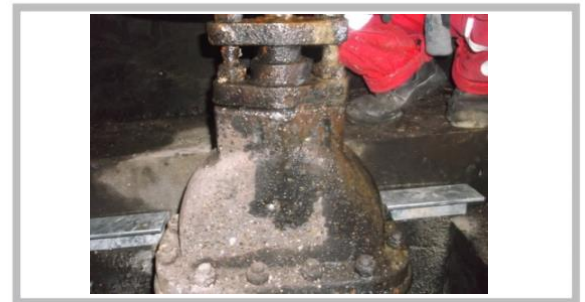
Gate Valve Before Application
