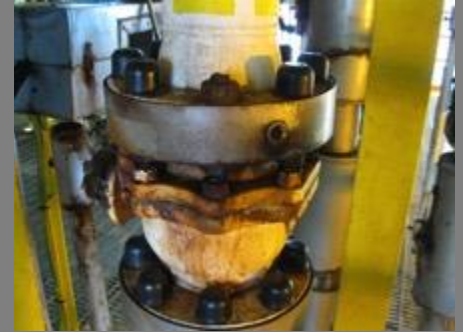
Note the use of plastic caps has failed and not possible to apply to all bolts and nuts
